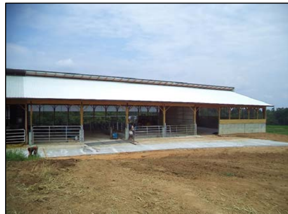
[After] Completion of Animal Heavy Use Area and 60' x 40' x 6' dry stack manure storage. Storage provides 4-6 mo. Capacity
