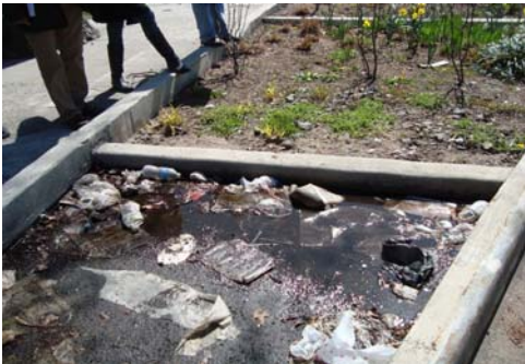
Curb Check Dam Causing Urban Trash Eyesore
