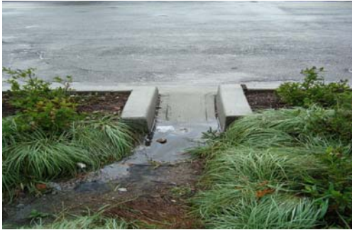
Oil and Grease entering Rain Garden Without Pretreatment
