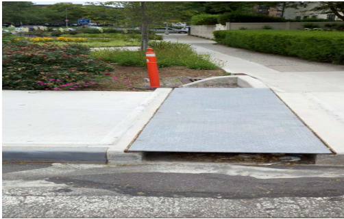
Trash Entering Rain Garden or Causing Back Up
