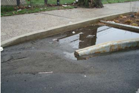
Ponding of Water at Entry to Rain Garden
