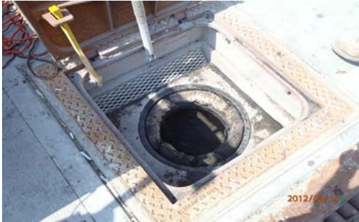
Terre Urban Protector after Maintenance 1 Man Hour for Maintenance
