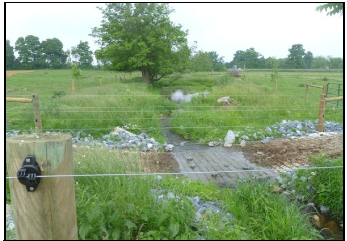
This "After" picture shows the stream crossing several months after construction providing buffer.
